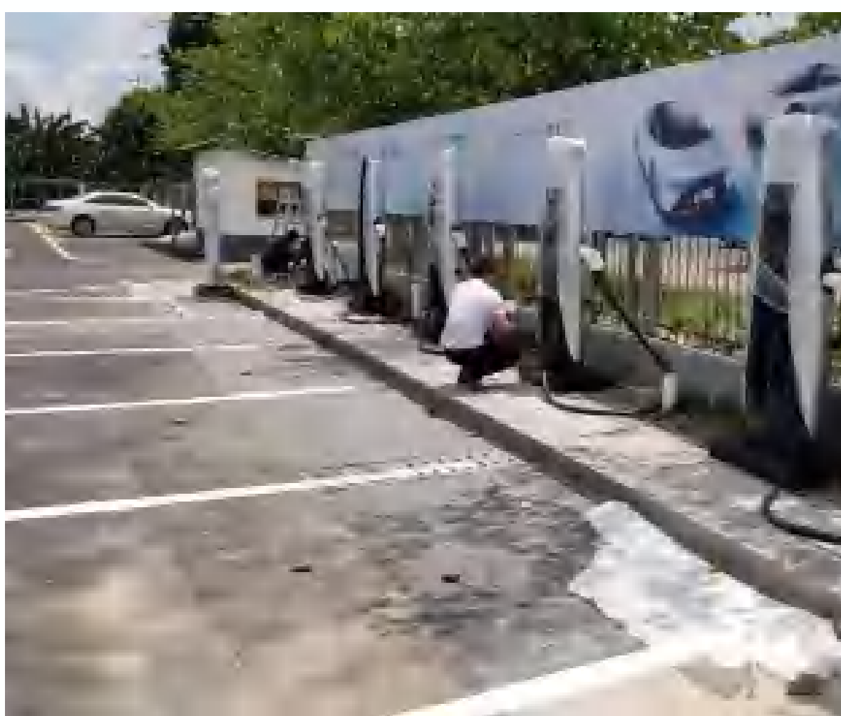
Aion Super Fast Charging Station Case
