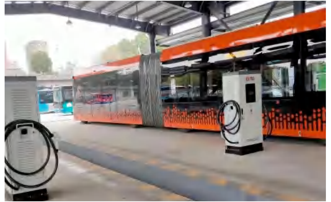
Rail Car Charging Station Case
